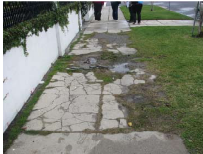
Broken & Missing Sidewalk Segments
