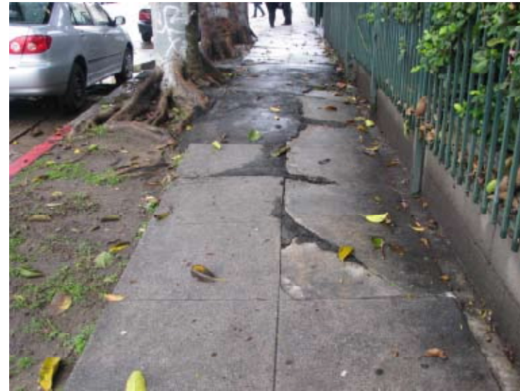
Trees Cracking Sidewalks
