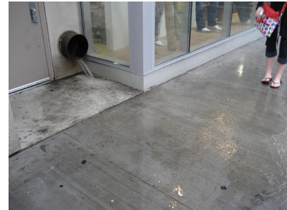
Figure 16 - Stormwater runoff from commercial properties on Western Avenue flowing directly onto the pedestrian pathway
