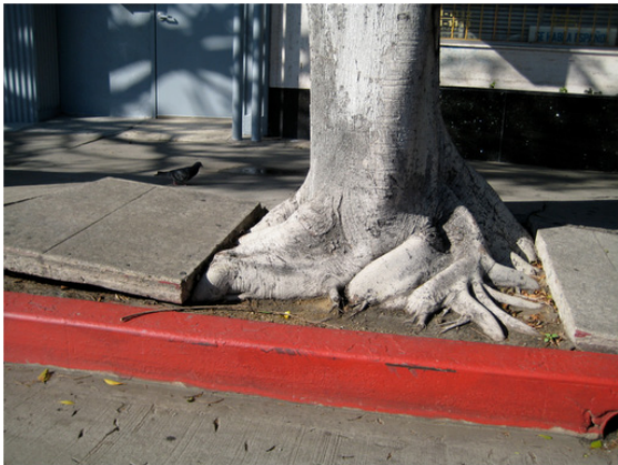
Figure 17 - Cracked sidewalks along 8th Street
